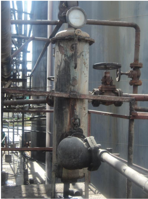
Flash steam recovery unit
